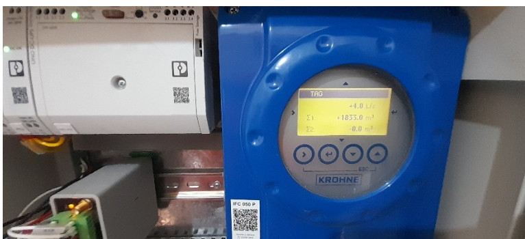
Vista interior do painel
