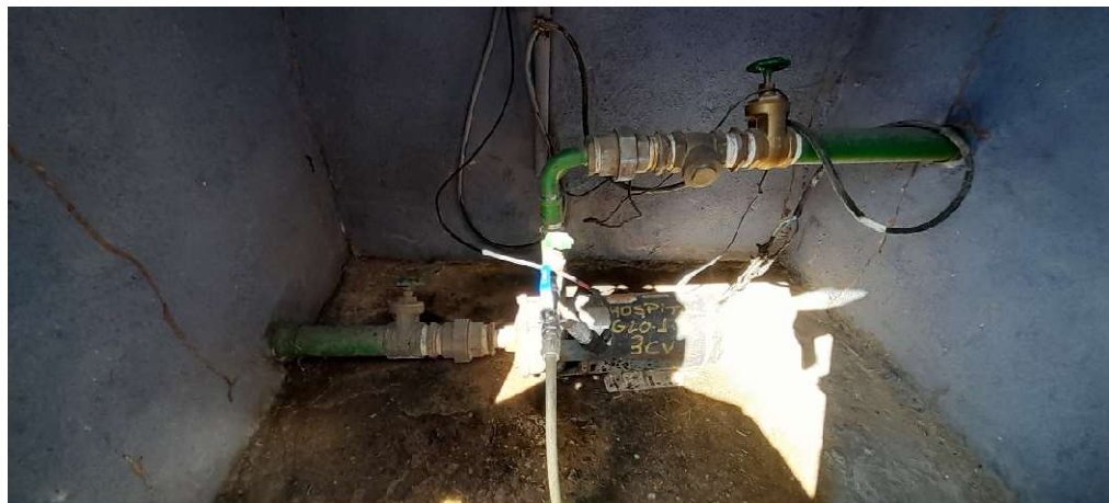
Eletrobomba booster do Hospital
