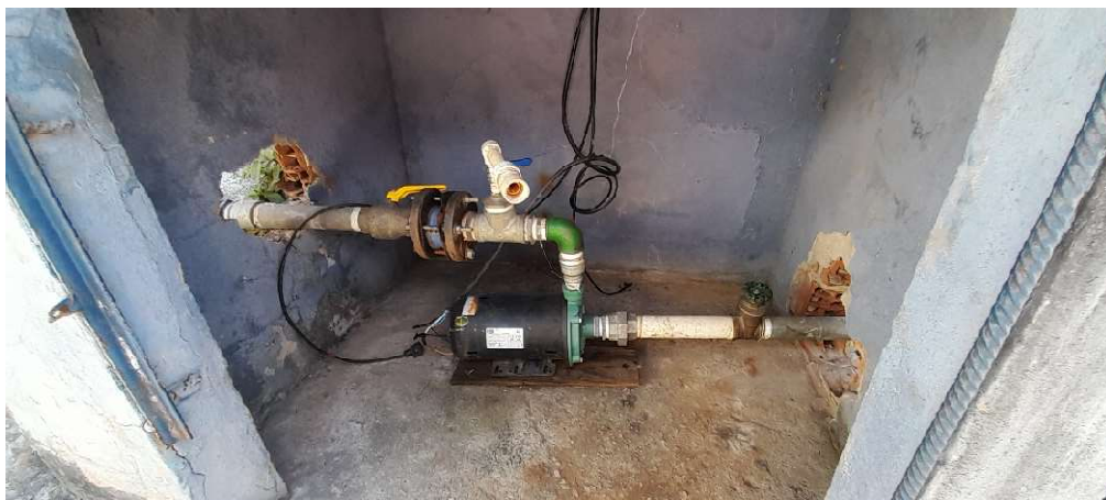
Eletrobomba Francisco Guida
