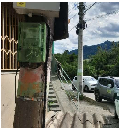
Booster e Painel de Controle do CCO
