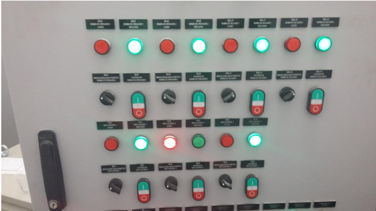
PAINEL DE CONTROLE
