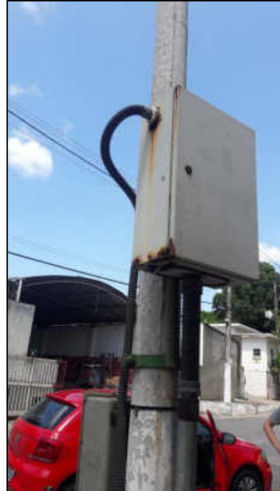
Painel de controle
